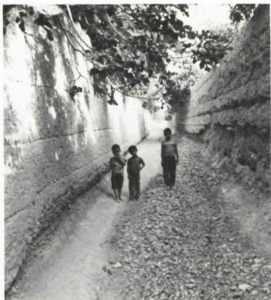
FIG. 14. Erosion of walls by a water channel in Mehriz.
